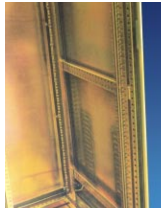
Louvres for airflow are backed by perforated grill
